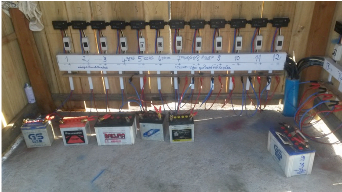
Figure 1. An example of under-utilized battery charging station
