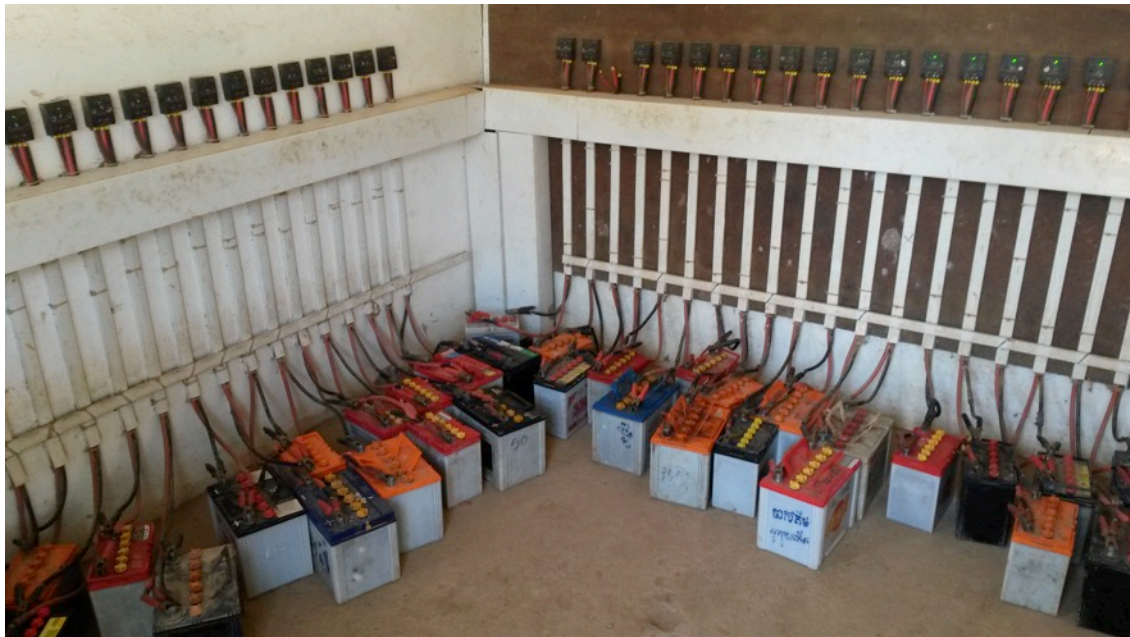
Figure 3. All types of batteries of different capacities being charged (faulty charge controllers not replaced due to lack of technical personnel)
